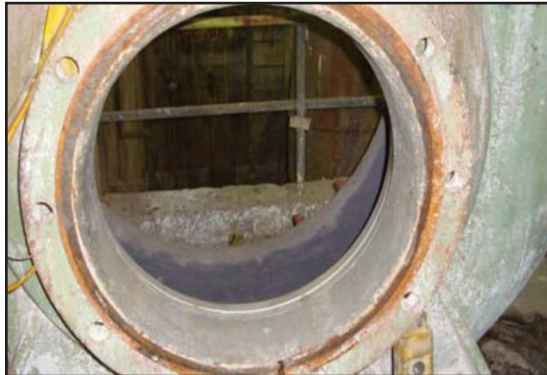
Damaged pump casing
